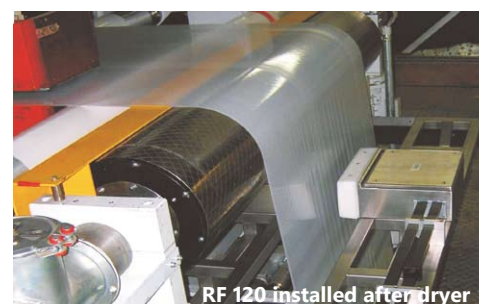
RF 120 installed after dryer
